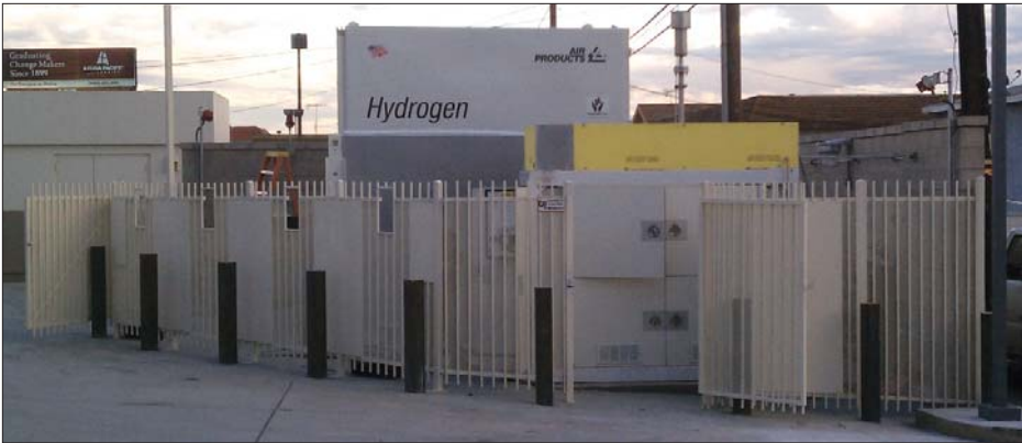
The key to the cost effective “compression-less hydrogen fueling station” is a composite pressure vessel (CPV) trailer as pictured in this photo. The trailer containing the CPVs and associated equipment inside the fenced area are located in the corner of the forecourt space of an existing retail gasoline station in California. Underground piping directly supplies the hydrogen to the fuel dispensing equipment.
